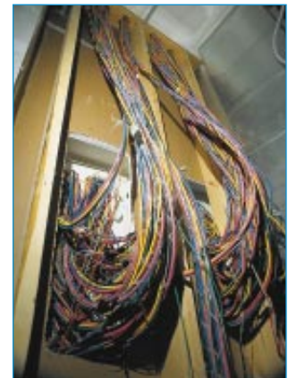
NETWORK CABLE: about 10 miles' worth in total.
